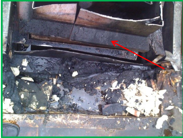
Arrow pointing to wood blocking around hot ductwork
